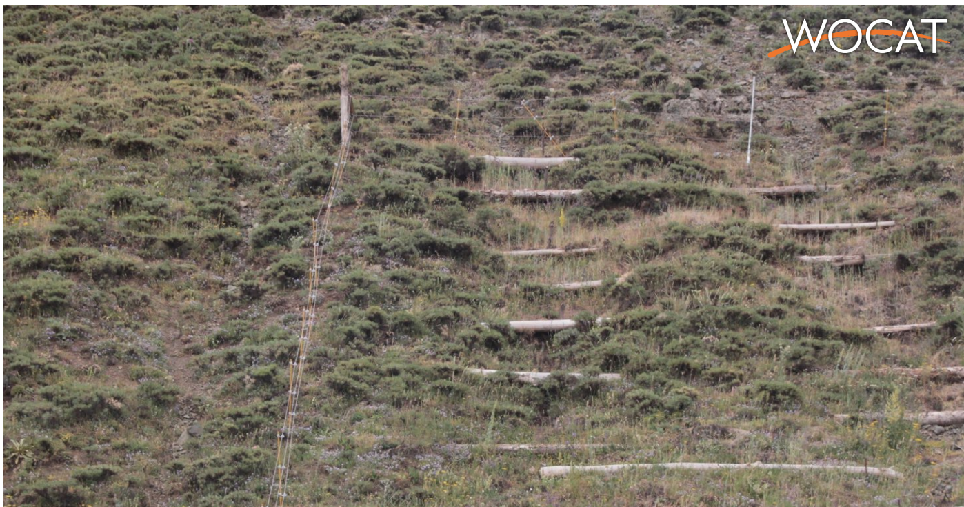
Pilewalls with additional mulch cover after 6 months; Protection by electric fence against grazing (Huber, M.)
